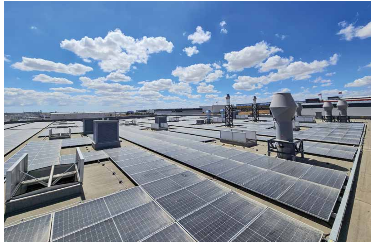
View of the photovoltaic system on the production building at the EJOT site in Çerkezköy, Turkey.
