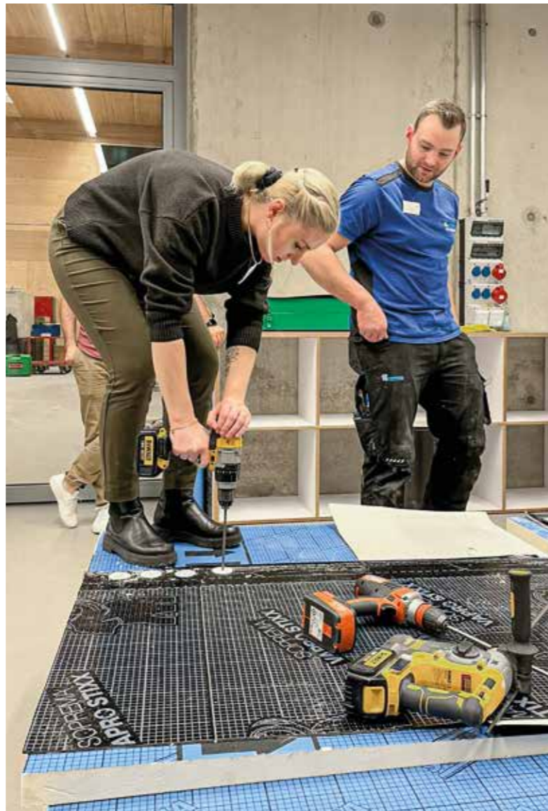
The face-to-face events involve a lot of hands-on work, as can be seen here at our focus day on flat roofs with Soprema.
