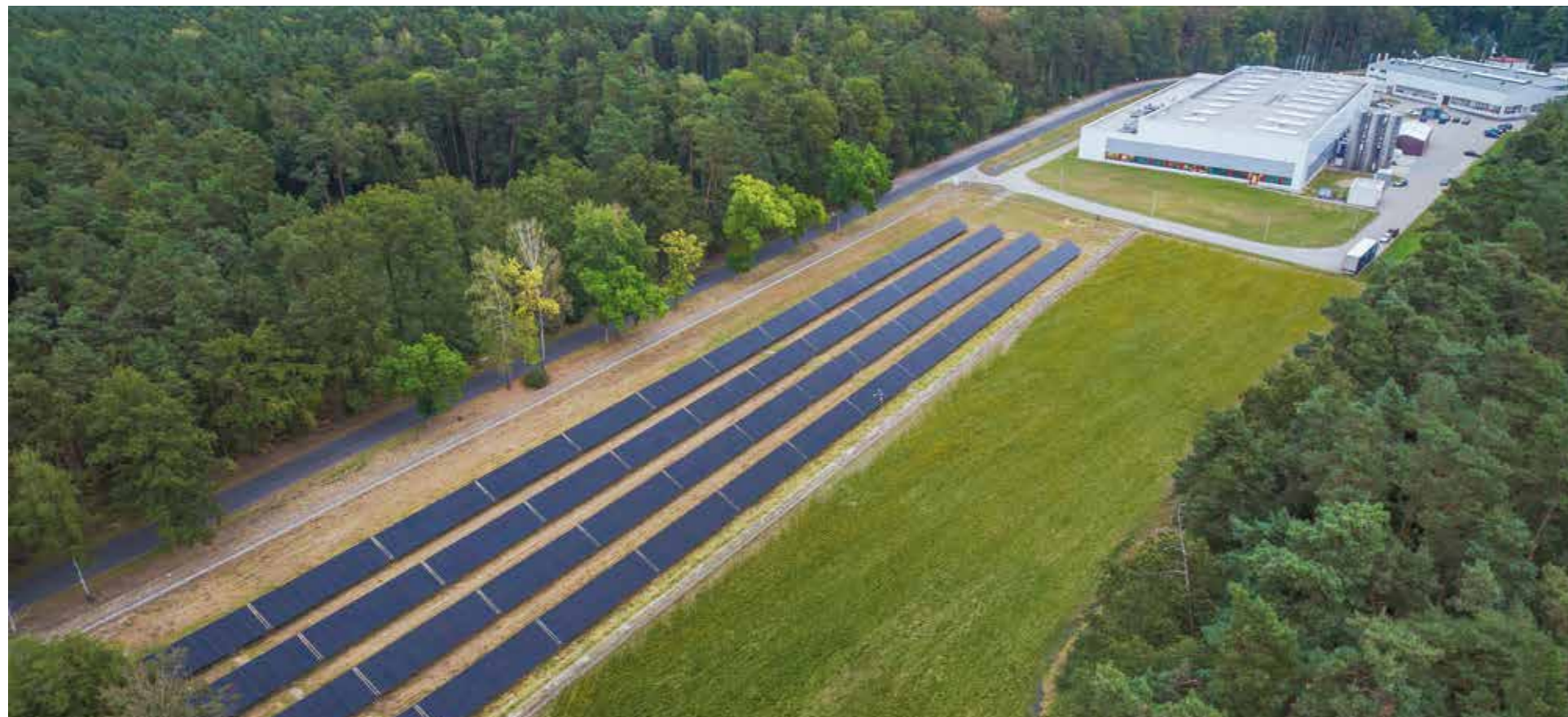
The new photovoltaic system at the EJOT site in Ciasna, Poland has been in operation since September.
