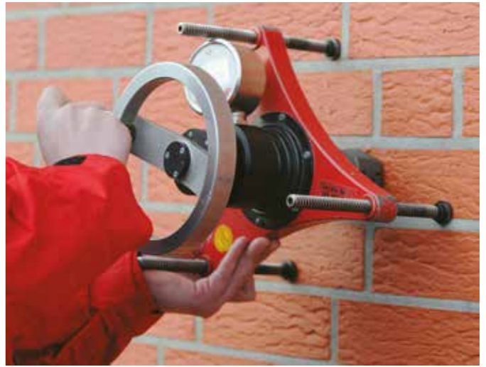
Anchor pull-out tests at the construction site to determine the right fastener
